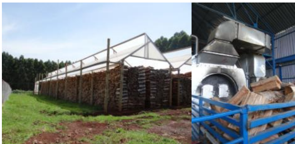
Figure 20: Firewood stock under greenhouses for drying and boiler fed by woody biomass at Finlays estate (Kericho)
